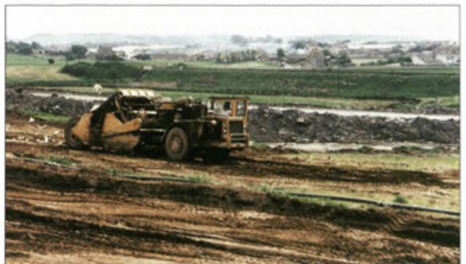
Figure 1. A box scraper stripping the topsoil at an opencast coal site. (Photo: SOAFD)
